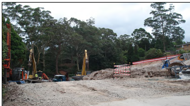
Blue Gum High Forest site is moonscaped by damage un-assessed under one LEP, while damage from an adjacent development is cumulatively allowed under another LEP.
