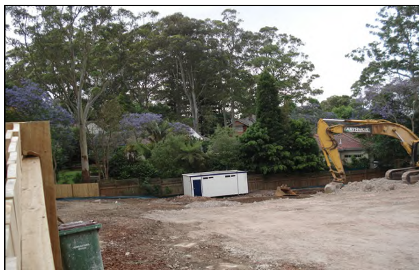
As sites are cumulatively cleared, the very basis for fragile Urban Forest ie. rich soils and seed-bank, is excavated and removed forever by improper planning.
